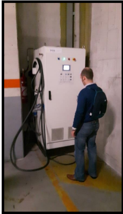
Electric charging unit
